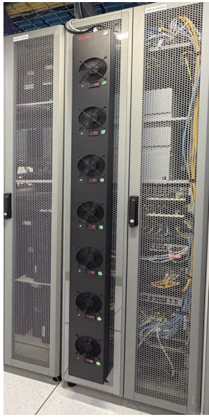
Smart Fan Unit – Slave (OIF-F7S-1) Front door 7 fans – intake airflow
