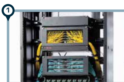
CABINETS/ POWER DISTRIBUTION UNITS/ KVM SWITCHES/ SLIDING SHELVES
